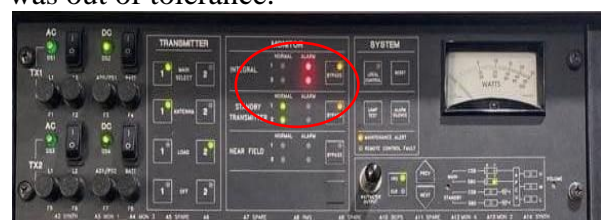
Figure 2. Alarm Condition on Monitor LCU
