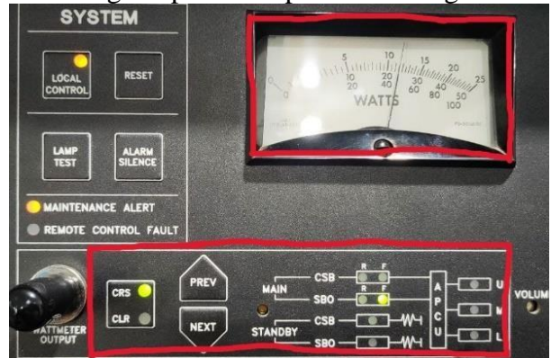
Figure 14. Wattmeter Power SBO Forward Reading Normal
