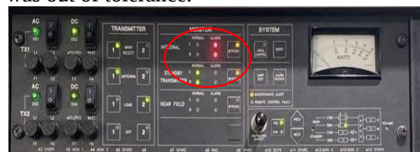
Figure 2. Alarm Condition on Monitor LCU
