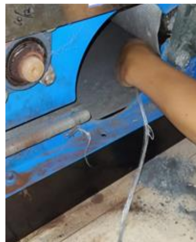
Figure 7. Cutting the damaged part of the Belt
